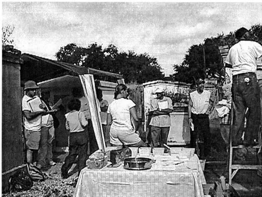
Above, workshop participants watch as Royal Osborne (on ladder) applies stucco to a tomb.
